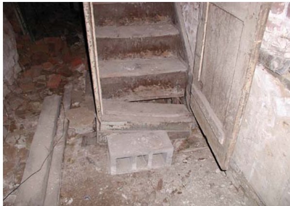
Removal of the historic floor and deterioration of the stringers have left the bottom of the stair to the cellar unsupported and precarious.
