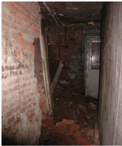
The south end of the brick stiffening wall between the cellar hall (B03) and the former kitchen (B02) has suffered partial collapse.
