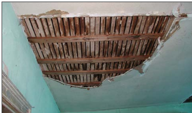
Figure 101: In Room 202 all of the original ceiling plaster was removed and a gypsum wallboard ceiling was installed on furring strips attached to original lath.
