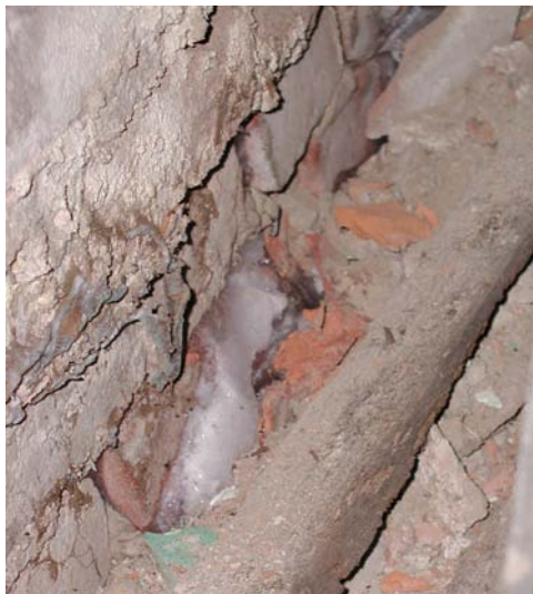
During a winter visit, ice was visible in the bricks in the east-west cellar partition.
