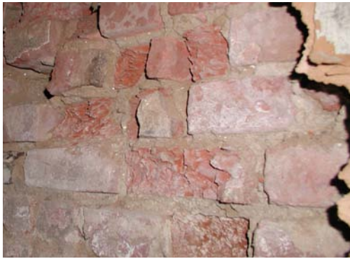
Repeat freeze and thaw cycles have left the bricks in the cellar walls brittle and friable.
