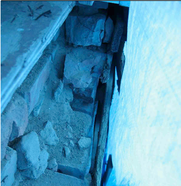
Photograph No. 13. View of the exterior brick below a second floor window sill (on the south elevation).
