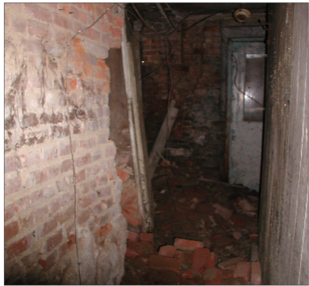
Figure 53: The south end of the brick stiffening wall between the basement hall (B03) and the former kitchen (B02) has suffered partial collapse.
