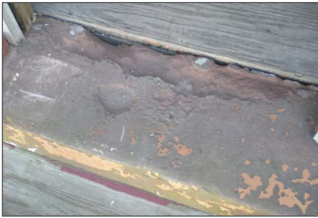
Figure 138: Deteriorated sandstone sill on the main entrance door will need restoration through limited patching.
