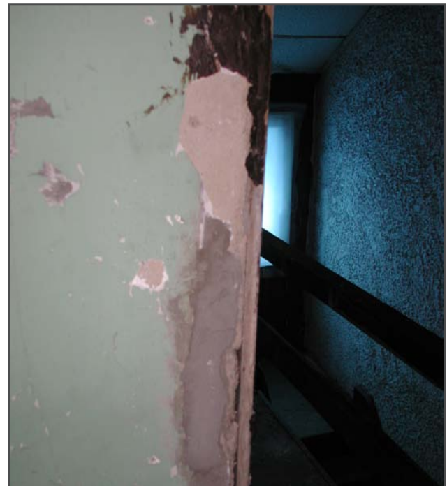
Figure 127: Damage to the outside corner in Room 304 exposed a wood corner bead.
