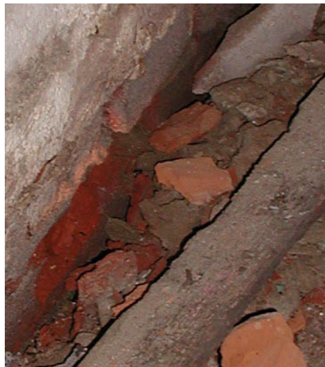
During a spring visit, damage was visible in the bricks in the east-west cellar partition, where the ice has melted.
