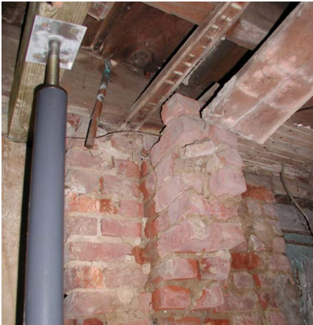
Figure 136: Lally columns in the basement are temporarily supporting the collapsing stiffening wall, but shoring, bracing and reconstruction of this wall are needed to sustain the building's structural integrity.
