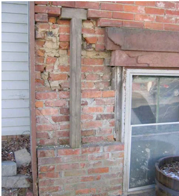
Photograph No. 17. View of localized failure of exterior wythes of brick masonry at the NE corner of the building.
