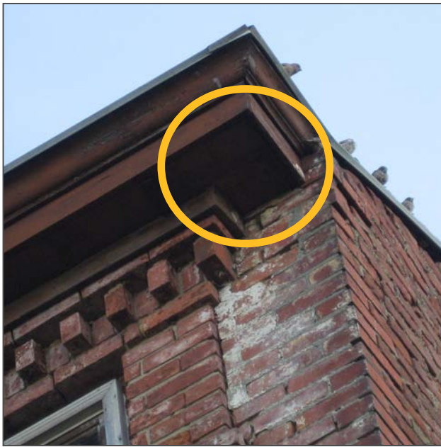
Figure 37: North facade cornice at the corner of the west facade with a detail of the failing built-in gutter system. The location of a since-removed leader is highlighted.
