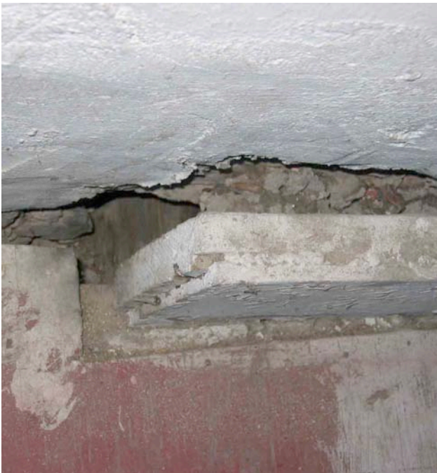
Photograph No. 15. View of another landing of the main staircase where the header and the stair have moved away from the interior face of the exterior wall.
