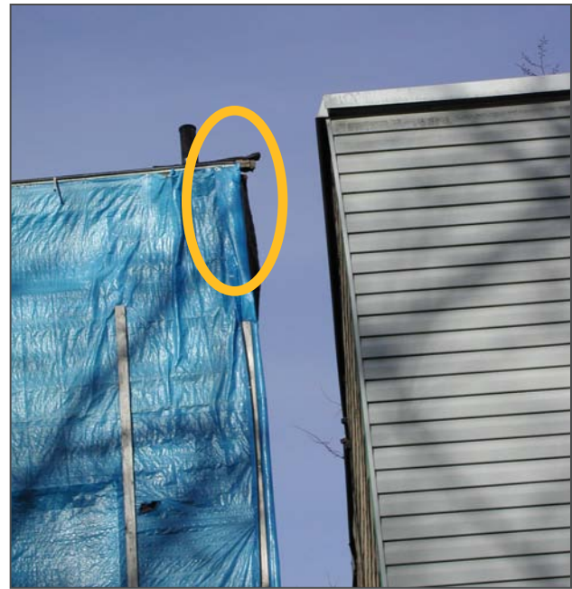
Figure 49: View from rear (south). The masonry at the upper portion of the gable on the east façade is visibly bulging.
