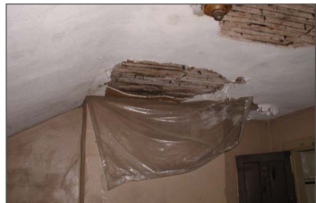
Figure 118: Damage to the plaster ceiling along the east wall in Room 301 was likely caused by water entering through failed chimney flashings.
