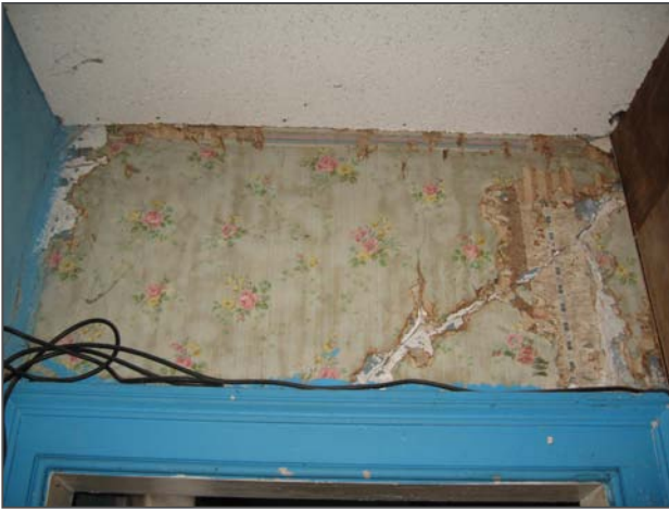
Figure 113: Layers of wallpaper visible over the door trim on the eastern wall.
