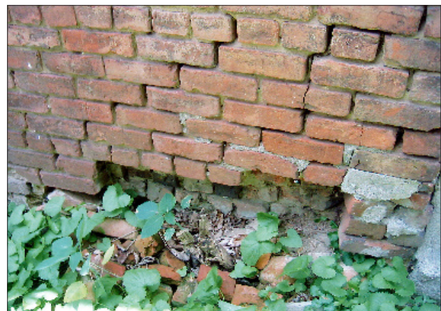
Figure 42: Weakened masonry at the south end of the west façade (note severely eroded mortar joints) has partially collapsed.
