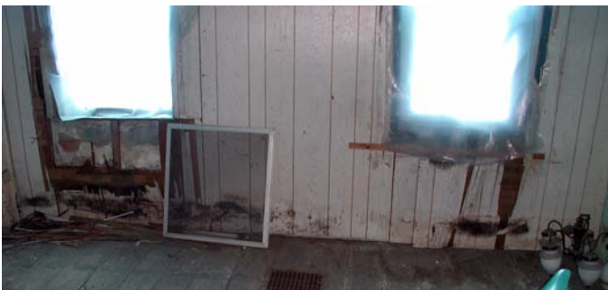
Ongoing water infiltration through the south wall of Room 202 has damaged both the original plaster wall finish and the faux wood paneling installed to hide the ruined plaster.
