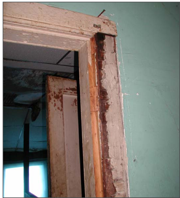
Figure 133: A missing door casing in Room 306 reveals that the lath and plaster base coat continued behind the trim. The final coat of plaster was installed after the casing was in place.
