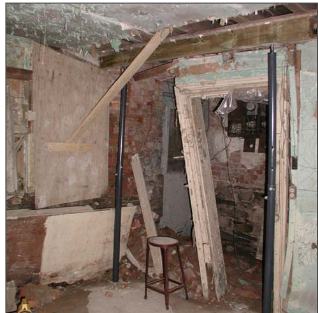
Figure 65: Ongoing water infiltration has destroyed many of the finishes in Room B02.
