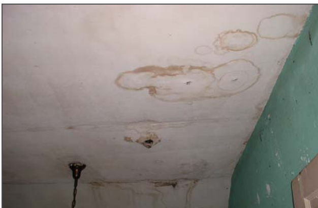
Figure 132: Water damage is clearly visible on the ceiling of Room 306.
