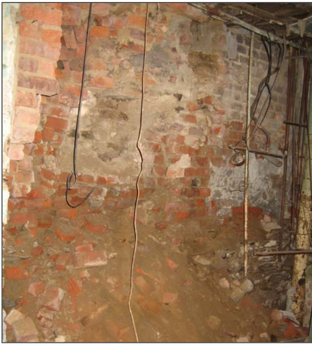
Figure 67: Collapsed chimney breast on the east wall.
