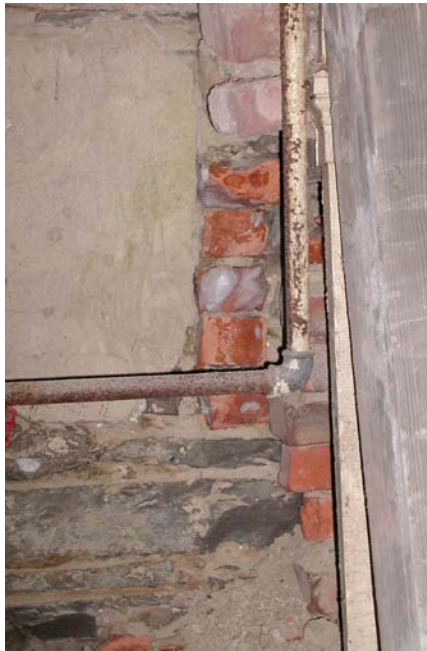
This iron pipe in Room B01 was most likely a gas pipe.
