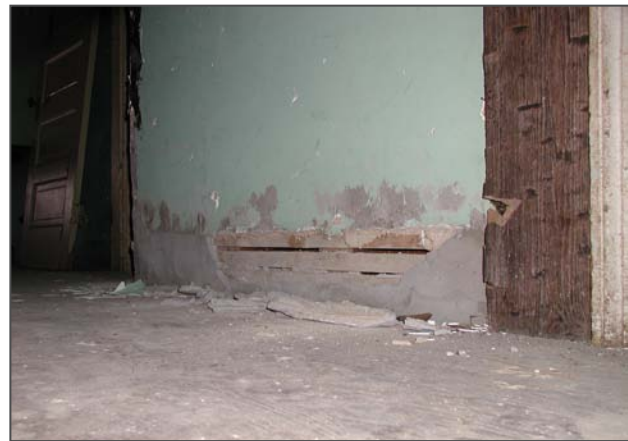
Figure 124: In Room 304, the baseboards were removed and the exposed space parged with cement.
