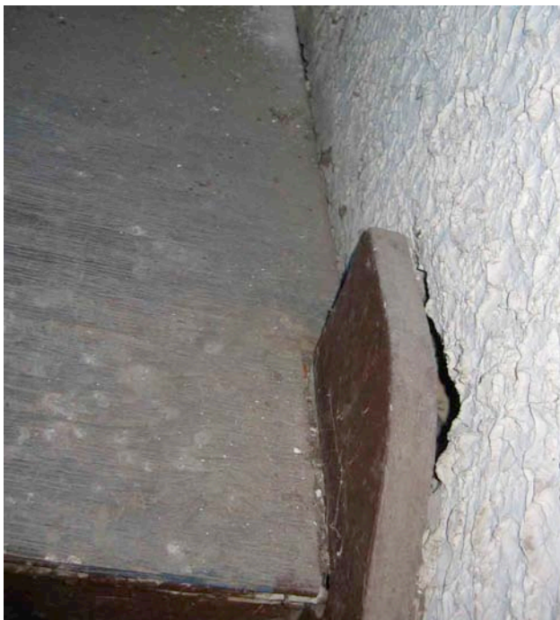
Photograph No. 11. View of stair landing at upper floor where the stair has pulled away from the interior surface of the exterior wall.
