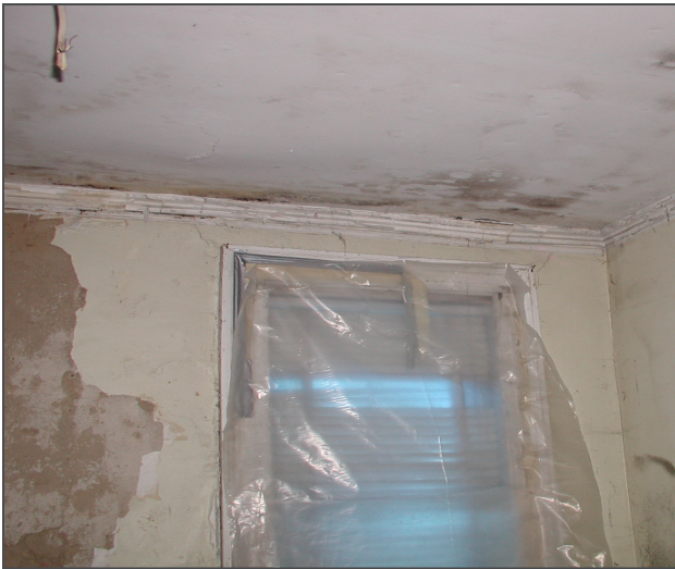
Figure 79: Water infiltration through the south wall damaged the plaster walls and cornice and left mildew stains on the ceiling of Room 102.
