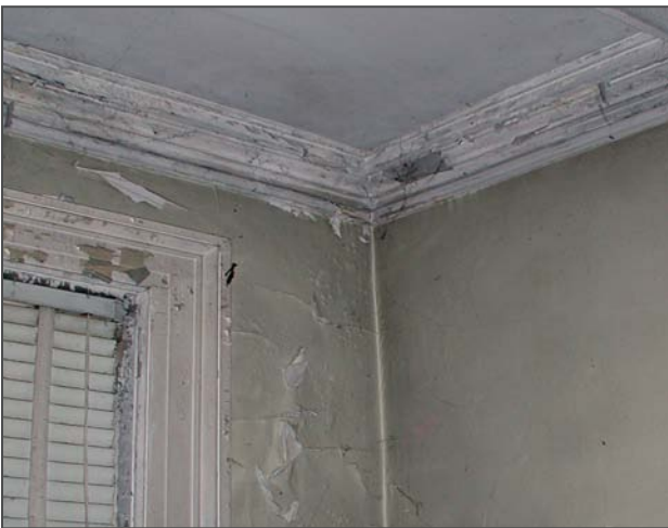
Figure 74: In the northeast corner of Room 101, peeling paint and soft plaster indicate moisture infiltration.
