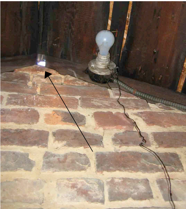
Photograph No. 16. View of interior surface of the west gable as viewed from the attic. The arrow points to where light (and water) enters the attic.
