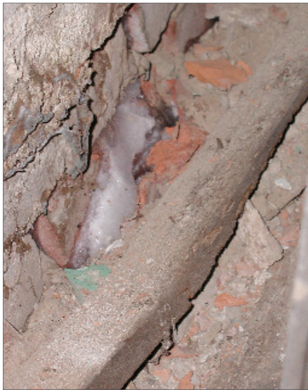
Figure 56: During a winter visit, ice was visible in the bricks in the east-west basement partition.
