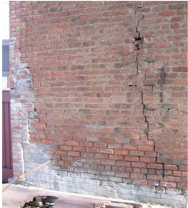
Photograph No. 20. View of one of the cracks in the masonry at the base of the West elevation wall (near NW corner of the building).
