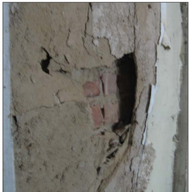
Figure 78: Southern wall in Room 102 in between the windows. Severe water infiltration has resulted in the plaster detaching from the brick, buckling and falling off.
