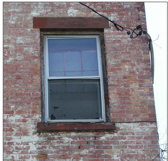
Figure 35: Door and window openings on the north façade are accented with reddish-brown sandstone lintels and sills.
