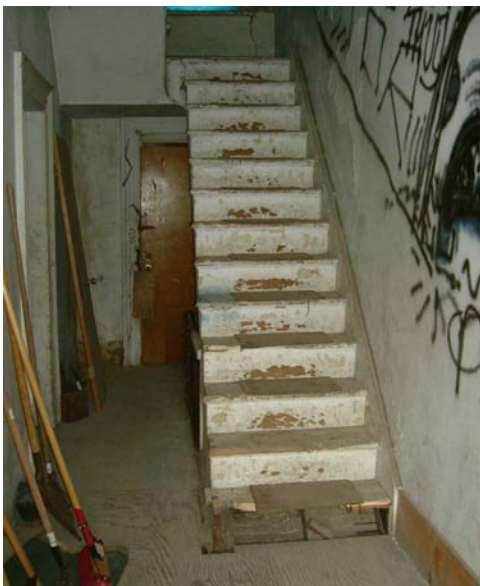
Stairs at first floor require a railing and should not be used by public.
