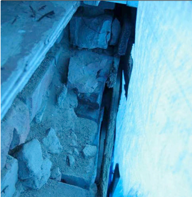
Photograph No. 13. View of the exterior brick below a second floor window sill (on the south elevation).
