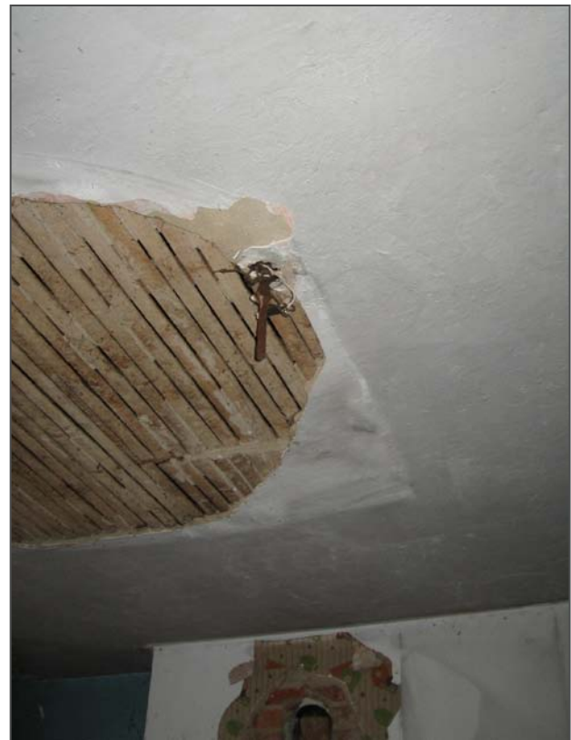
Figure 95: Remnants of an electrical fixture on the ceiling next to a large section of broken plaster.
