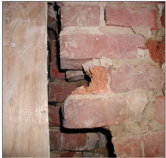
Figure 137: Water infiltration in the basement has severely damaged numerous bricks beyond the point of repair.
