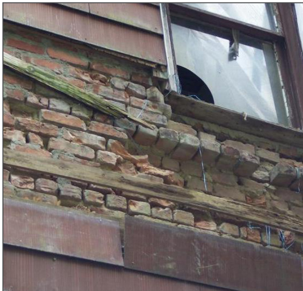
Figure 45: When a new tarp was added to the south facade in June of 2008, fallen asbestos siding revealed the deteriorated masonry wall underneath.
