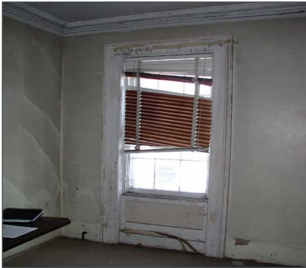
Figure 73: In Room 101, the front parlor has the most elaborate finishes in the house: a run plaster cornice and recessed wood panels below the windows. Diagonal cracks (at left in this photo) indicate settling.
