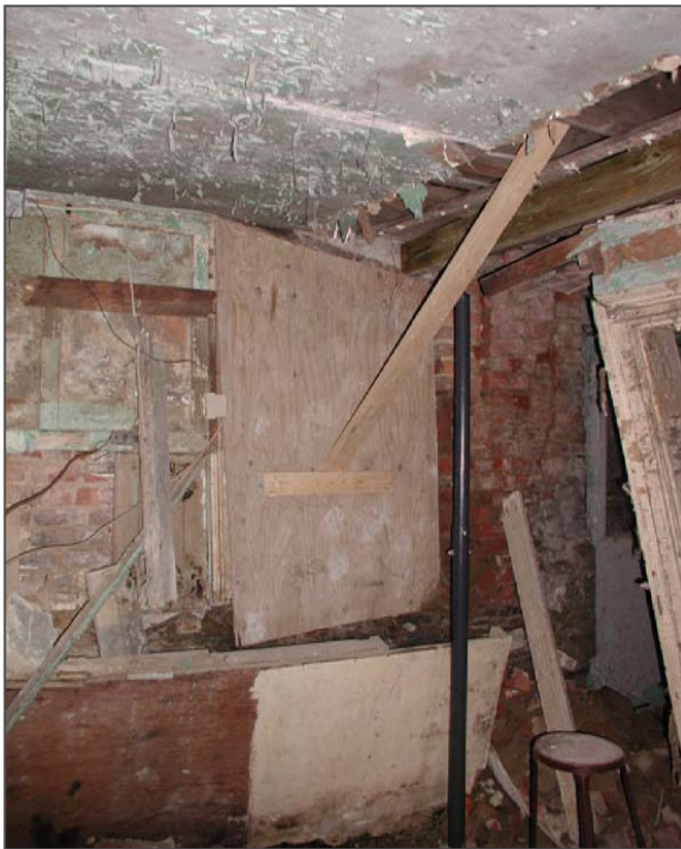
Figure 52: All of the brickwork at the south end of the stiffening partition between B02 and B03 has collapsed. Temporary posts and beam support the first floor.
