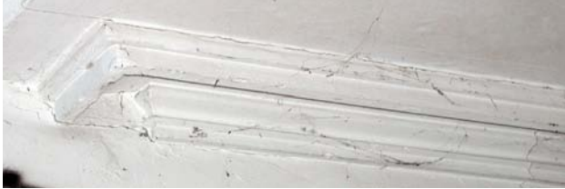
Room 103 retains an original plaster cornice. This cornice should be supported and protected from damage during the Stabilization work.
