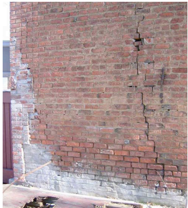
Photograph No. 20. View of one of the cracks in the masonry at the base of the West elevation wall (near NW corner of the building).
