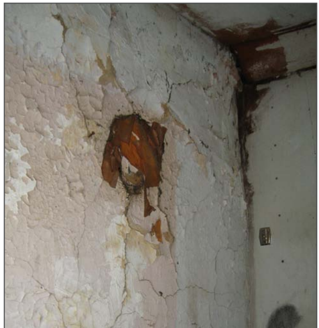
Figure 135: Former location of a stove hole in the chimney breast on the east wall of Room 302 is evidence of an original or early use of a stove to heat this space.
