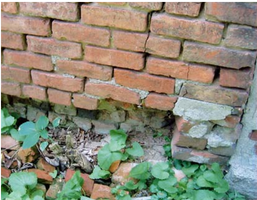
Weakened masonry at the south end of the west façade (note severely eroded mortar joints) has partially collapsed.
