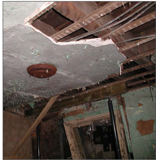
Figure 64: Both plaster and lath are missing from the ceiling in B02.
