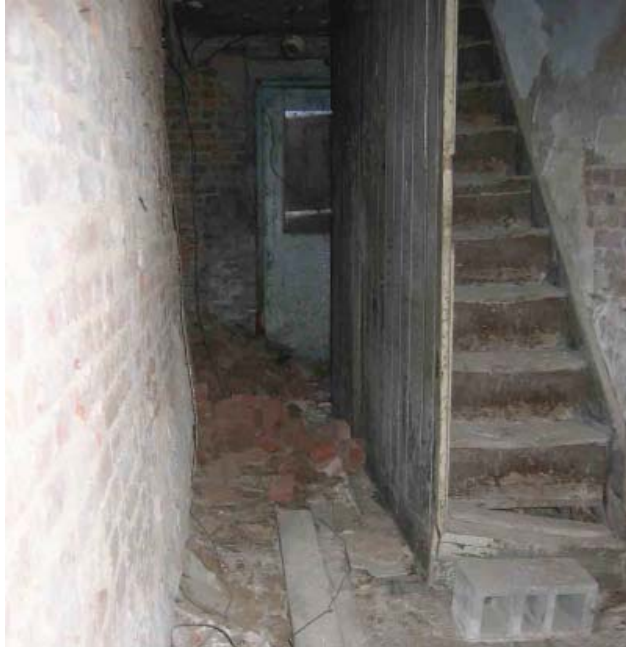
Photograph No. 9. View of basement hallway looking south. The north/ south bearing wall is on the left side of this image; note that the wall is no longer plumb and has moved sideways.
