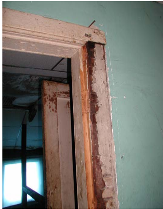
A missing door casing in Room 306 reveals that the lath and plaster base coat continued behind the trim. The final coat of plaster was installed after the casing was in place.
