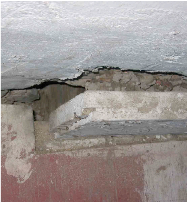
Photograph No. 15. View of another landing of the main staircase where the header and the stair have moved away from the interior face of the exterior wall.
