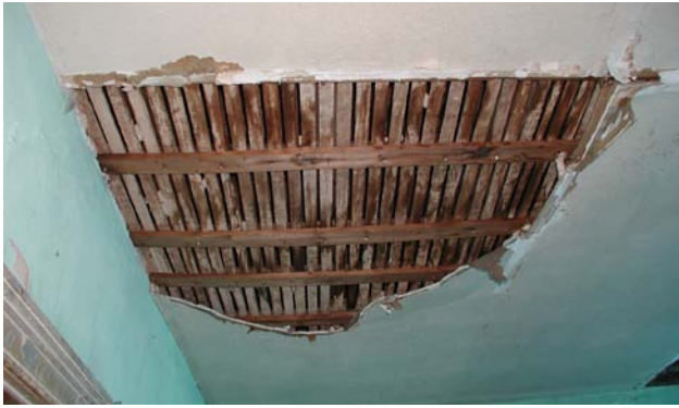
In Room 202 all of the original ceiling plaster was removed and a gypsum wallboard ceiling was installed on furring strips.
