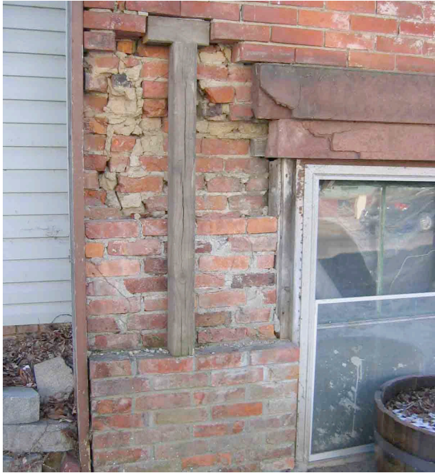
Photograph No. 17. View of localized failure of exterior wythes of brick masonry at the NE corner of the building.
