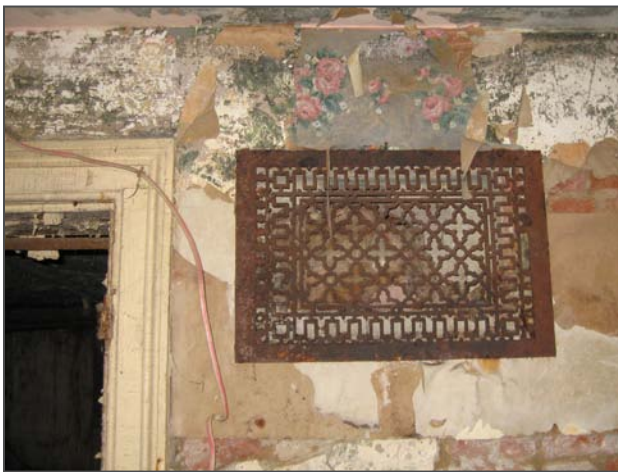
Figure 60: Cast iron grill on the south wall likely part of first central heating system.
