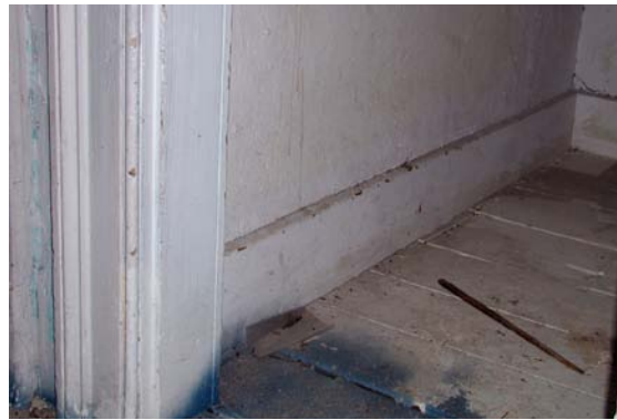
Room 204 is the only room in the entire house that retains original baseboards. The baseboard is a plain board with a beveled top edge.
