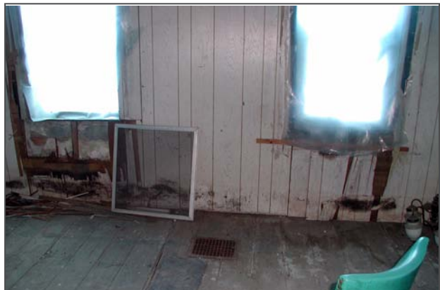
Figure 100: Ongoing water infiltration through the exterior south wall of Room 202 has damaged both the original plaster wall finish and the wood paneling likely installed to hide the ruined plaster.
