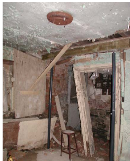
Ongoing water infiltration has destroyed many of the finishes in Room B02.
