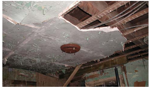
Both plaster and lath are missing from the ceiling in B02.
