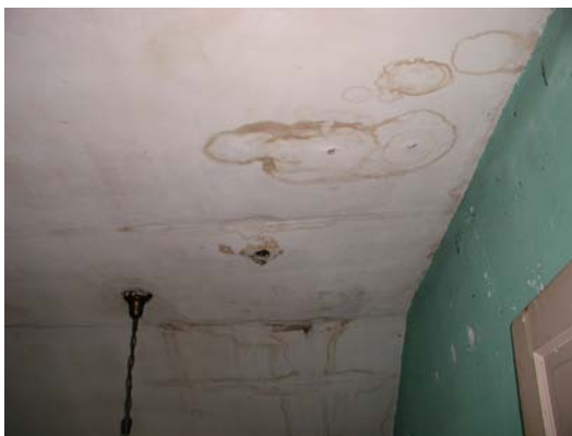
Water damage is clearly visible on the ceiling of Room 306.
