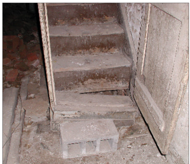
Figure 70: Removal of the historic floor and deterioration of the stringers have left the bottom of the stair to the basement unsupported and precarious.
