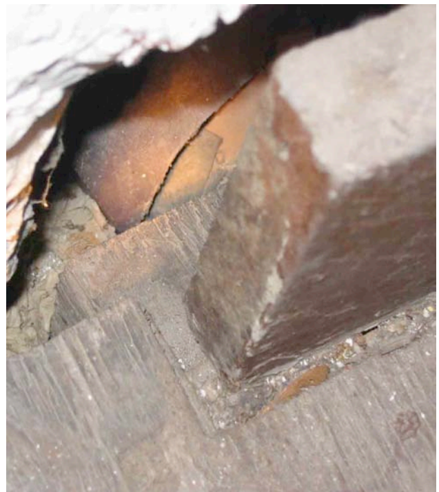
Photograph No. 12. View of header and side of stair landing at upper floor where the stair has pulled away from the interior surface of the exterior wall. This is a close-up of Photograph No. 11.
