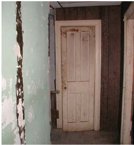
An original door frame with a four-panel, rail and stile door remains in place in the west wall of Room 304.
