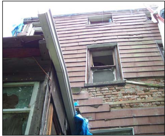
Figure 46: Exposed siding and brick on the south facade on June 20, 2008 when the tarp was being replaced.
