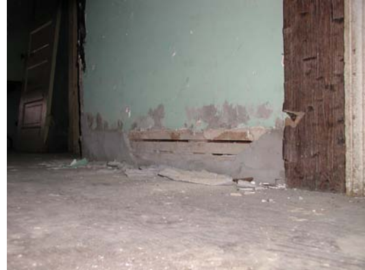
In Room 304, the baseboards were removed and the exposed space patched with cement.
