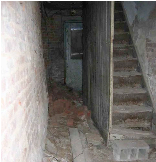
Photograph No. 9. View of basement hallway looking south. The north/ south bearing wall is on the left side of this image; note that the wall is no longer plumb and has moved sideways.
