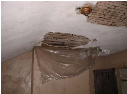
Damage to the plaster ceiling along the east wall in room 301 was likely caused by water entering through failed chimney flashings.
