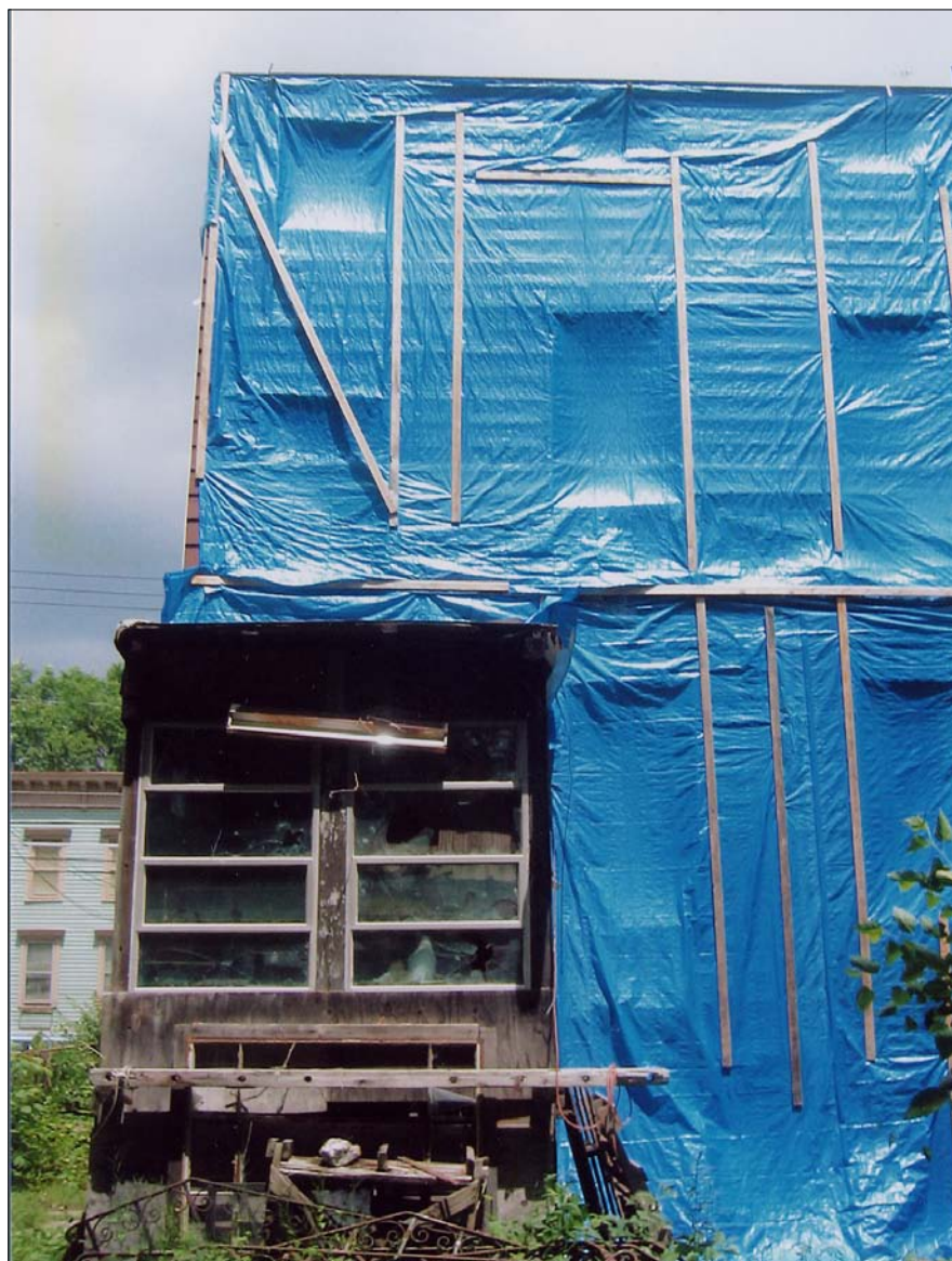
Figure 47: The south façade was covered in tarps to stop ongoing water infiltration during an initial attempt at stabilization in fall of 2004. The rear porch, a later addition, is probably not salvageable.
