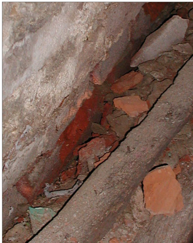
Figure 57: During a spring visit, damage was visible in the bricks in the east-west basement partition, where the ice has melted.
