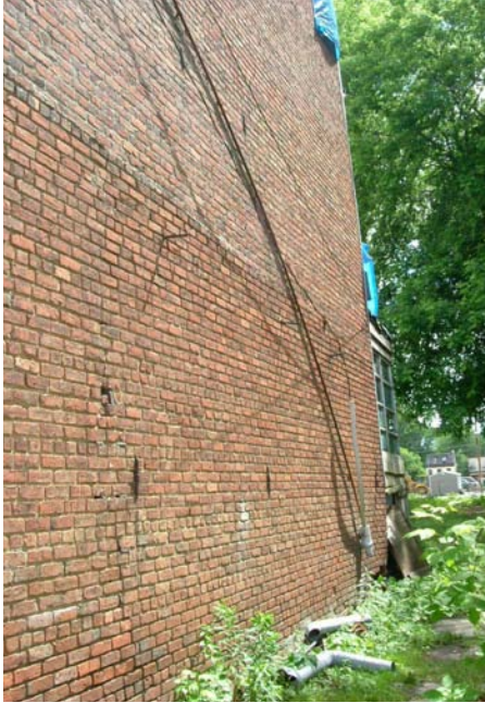
Wrought iron ties visible on the west façade strengthen the connection between the joists and the masonry.
