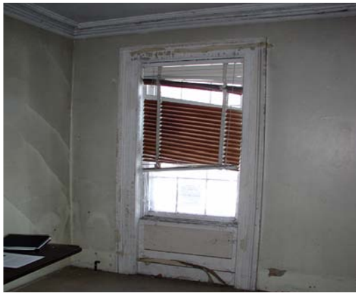
In Room 101, the front parlor has the most elaborate finishes in the house: a run plaster cornice and recessed wood panels below the windows. Diagonal cracks (at left in this photo) indicate settling.
