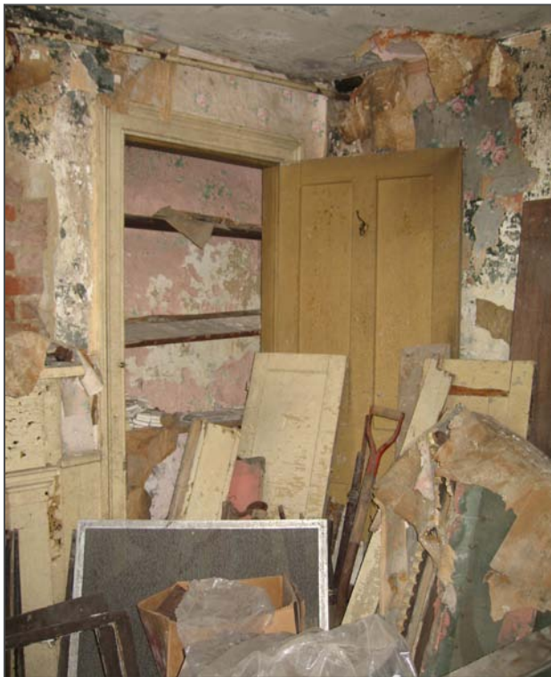
Figure 62: Closet and likely original door on the east wall in Room B01.
