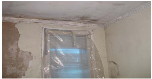
Water infiltration through the south wall damaged the plaster walls and cornice and left mildew stains on the ceiling of Room 102.
