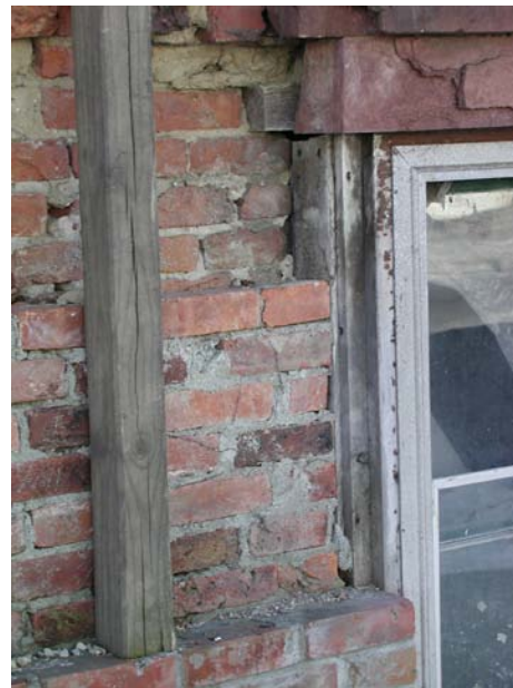
Brickwork at the east corner of the north façade has partially collapsed and requires immediate attention (note temporary support).
