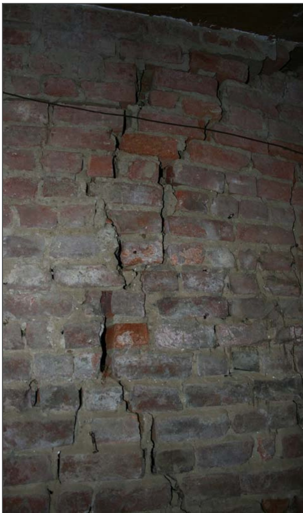
Figure 69: Large vertical crack in the stiffening wall.
