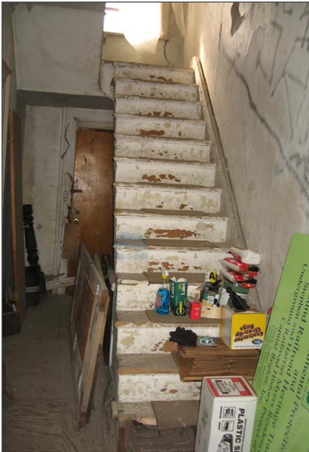
Figure 83: Staircase to the second floor with missing railing and balluster.
