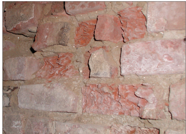
Figure 54: Repeat freeze and thaw cycles have left the bricks in the basement walls brittle and friable.
