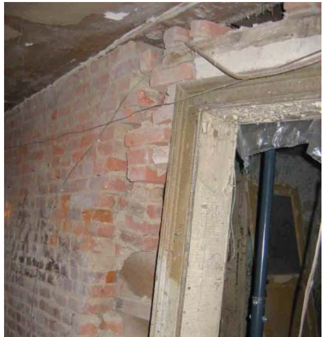
Photograph No. 4. View of the south end of the north/south bearing wall in the basement. Note the significant loss of bricks and disintegration of the wall.
