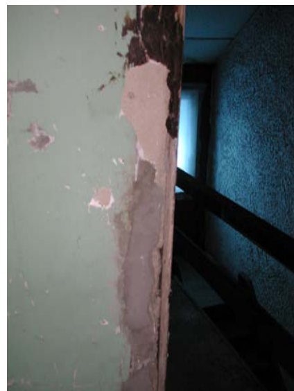
Damage to the outside corner in Room 304 exposed an original wood corner bead.
