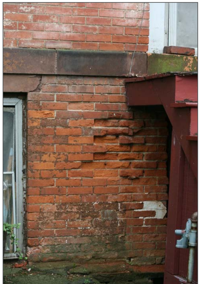
Figure 41: Area of spalling brick to the east of the contemporary stoop.
