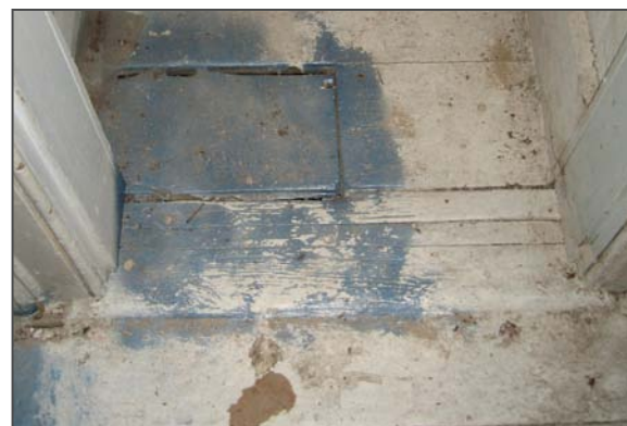
Figure 110: The east end of the floor has been cut, likely to facilitate access to the gas pipes serving the chandelier in Room 103 below.
