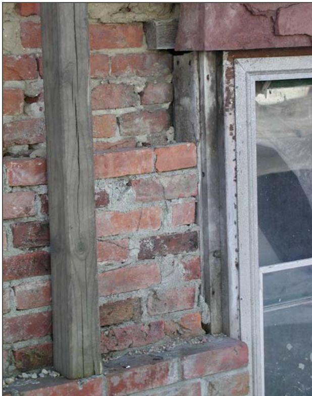
Figure 39: Two of three wythes of the brickwork at the east corner of the north façade have partially collapsed and require immediate attention (note temporary support).
