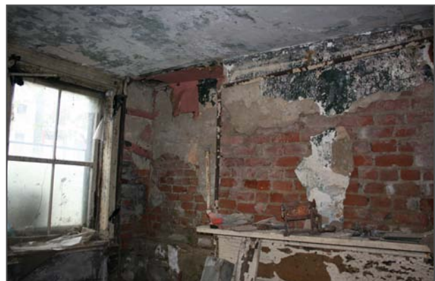
Figure 55: Most of the finishes in the basement are deteriorated from water infiltration. Plaster from the walls and chimney breast in the northeast corner of Room B01 have delaminated from the brick walls.
