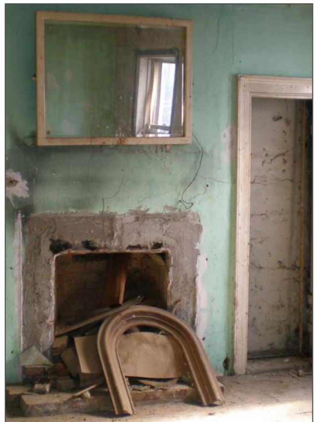
Figure 103: Room 202 has a shallow closet on either side of the fireplace opening. The mantelpiece was removed at an unknown date and the wall repaired with portland cement.
