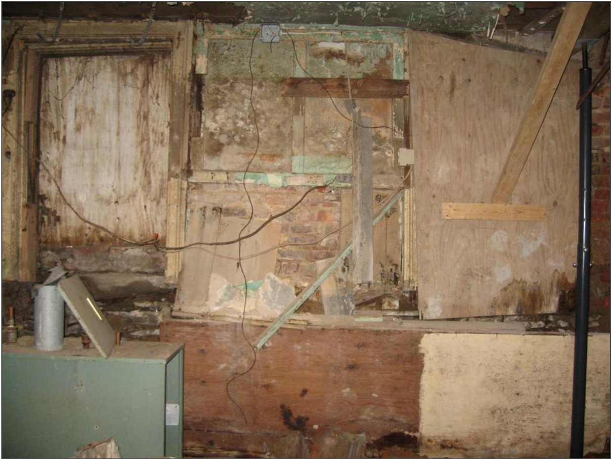
Figure 66: Boarded up windows on the south wall.
