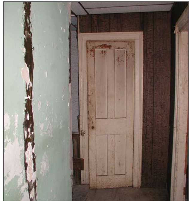
Figure 129: An original door frame with a four-panel, rail and stile door remains in place in the west wall of Room 304.
