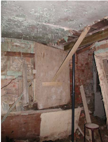
All of the brickwork at the south end of the stiffening partition between B02 and B03 has collapsed. Temporary posts and beam support the first floor.
