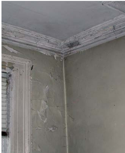
In the northeast corner of Room 101, peeling paint and soft plaster indicate moisture infiltration.
