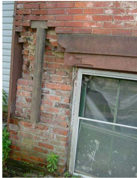
Missing bricks have left the northeast wall very thin and action should be taken immediately to reconstruct the wall.
