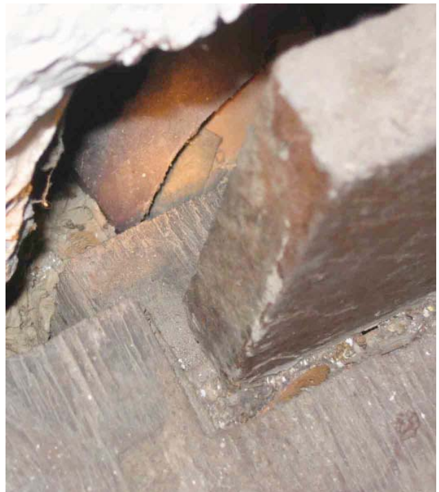
Photograph No. 12. View of header and side of stair landing at upper floor where the stair has pulled away from the interior surface of the exterior wall. This is a close-up of
