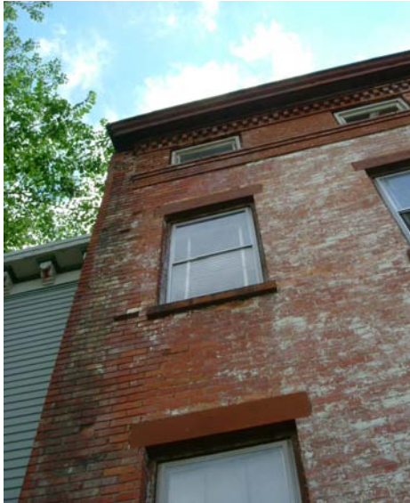
Stabilization of the exterior façades and structure must be completed before the Restoration work is begun.
